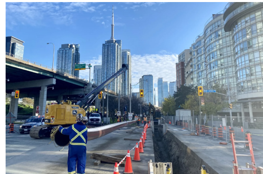
Helping Provide Natural Gas to the Citizens of Toronto Completed August 2023 | Toronto, Canada
